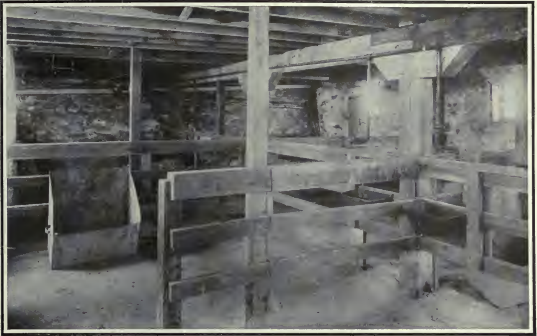
FIG. 257. HILLCREST DAIRY BARN (PIPING).
