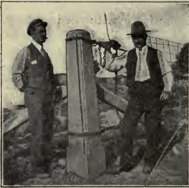
Figure 261. Stretching a ribbon of woven wire to attach it to a corner post.
