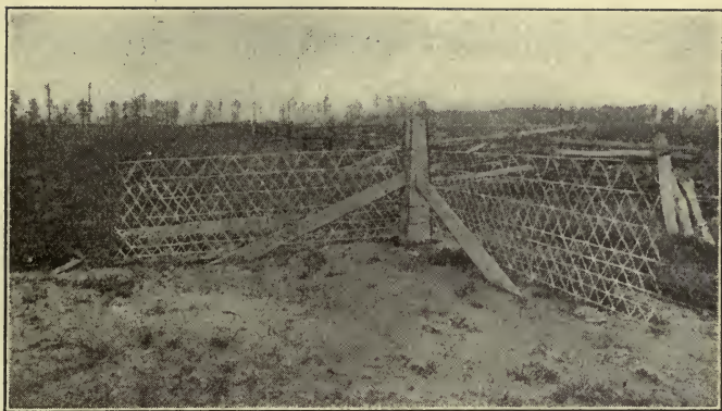
Figure 263. Cement corner post and braces, all made in place, for woven wire fence.
