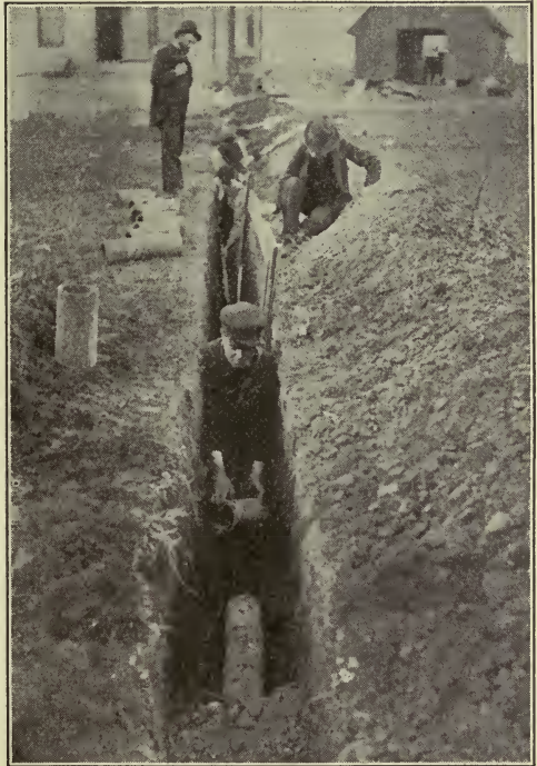
Figure 103. Agricultural high school students laying tile drains, showing how a man can get down into a narrow ditch.
