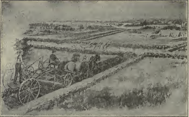
Figure 117. Reversible road machine making lateral ditches which run into a large drainage canal made beyond by the elevating grader.
