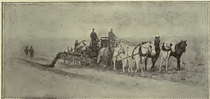
Figure 204. Elevating grader starting to plow out two roadside ditches and elevate the earth to the middle of the roadway.
