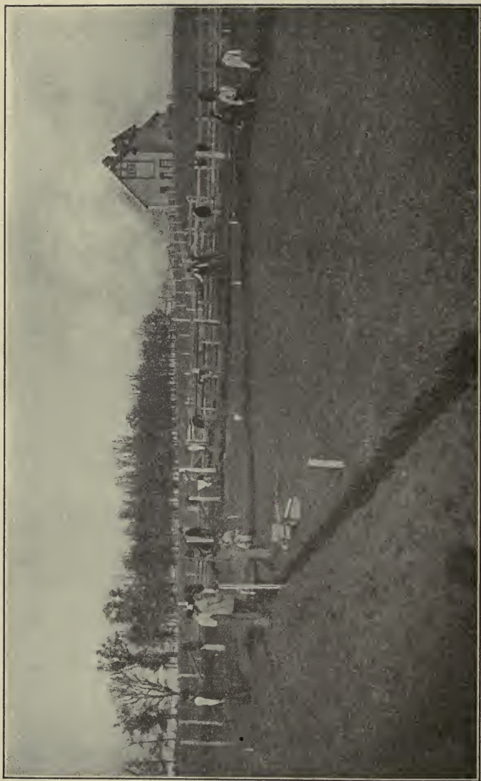
Figure 99. Students leveling bottom of tile ditch with device like that shown in Figure 96.
