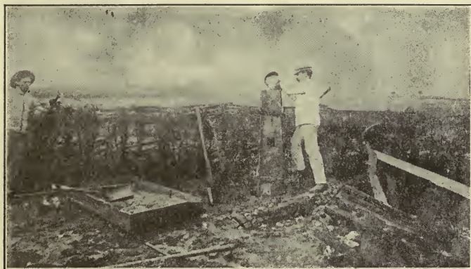
Figure 256. Filling the mold with cement after the wires have been placed inside. Hole left for the end of the brace mold.
