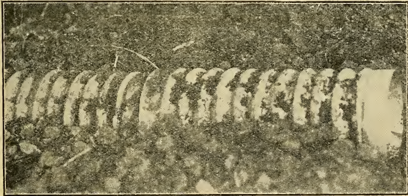
Plate 16. A corrugated steel culvert being poorly installed. Notice the lack of wing walls. The large clods are being dumped loosely about the culvert. The first heavy rain will probably wash out the culvert.
