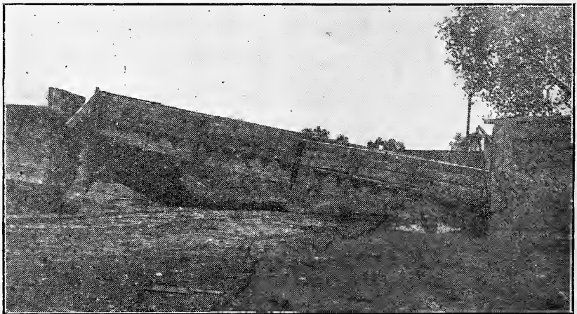
Plate 9. The large culvert or bridge shown in this plate had poor wooden wing walls which allowed the water to leak through and wash out the dirt back of the side walls. The "cave-in" came at the first heavy rain after the installation. Proper wing-walls and a proper tamping and puddling of the soil back of the side walls, would have made a good job out of a bad one.
