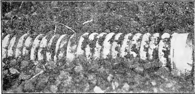
Plate 16. A corrugated steel culvert being poorly installed. Notice the lack of wing walls. The large clods are being dumped loosely about the culvert. The first heavy rain will probably wash out the culvert.
