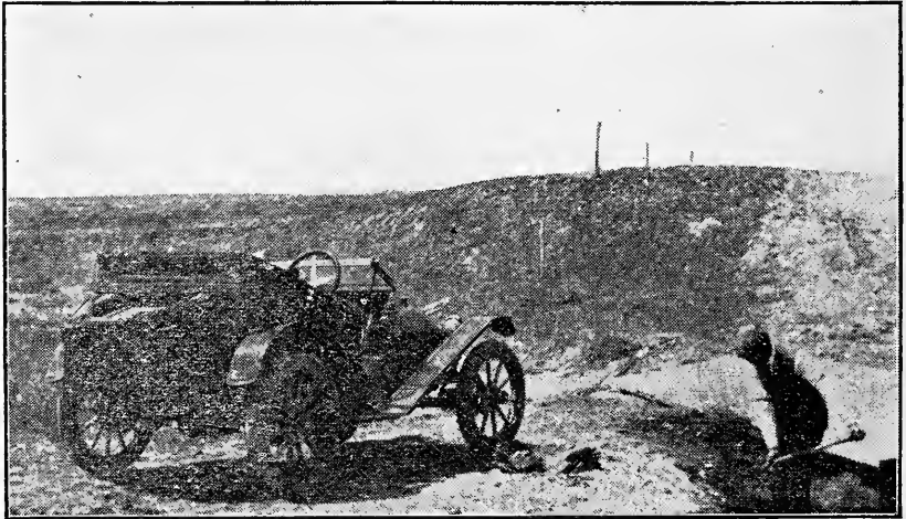
Plate 13. The culvert shown in Plate 13 was not protected by wing-walls. It was not tamped or puddled on the sides. A few days after the photo was taken, it was washed out and down stream.
