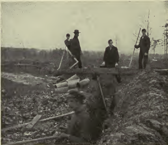
FIG. 40.—Laying drain tiles and testing the depth by measurement from level grade stakes.
