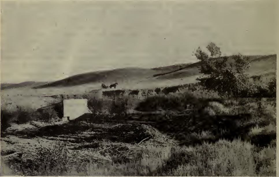
General view from down-stream side of rock and brush dam built across a creek. The dam is built up of alternate layers of brush and rock. The rock works down into the brush and so does not show up much in the photo. Note that the dam is started on a broad base and then gets narrower towards the top. This kind of dam is leaky until it gets filled up in front with mud and silt. This dam has flash boards placed on top of the crest but these are not necessary for the ordinary farmer's reservoir. This kind of dam is liable to be damaged if heavy ice comes down in the floods and is not as good as the wood and rock type of dam.
