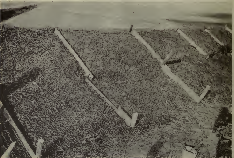
Close up view of an earth dam protected on the wet side with riprap made of straw held down with chicken wire and wood posts driven into the earth. Old boards have been nailed between the wood posts instead of using wire.
