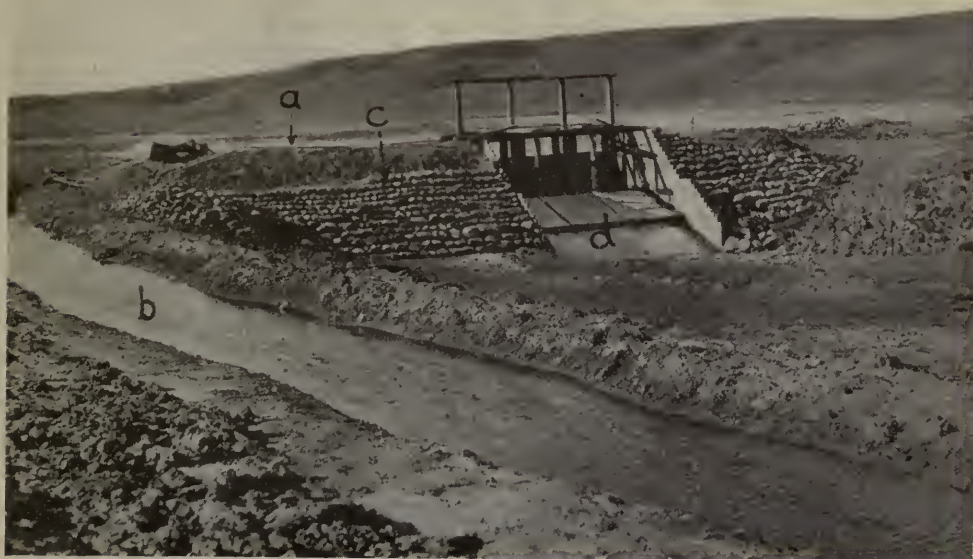
General view of earth dam. (a) Reservoir behind dam. (b) Ditch out of reservoir showing proper location for spillway channel around end of dam. (c) Rock riprap placed on dry side of dam to stop erosion by water running through wood spillway during floods. (d) Wood spillway through centre of dam. This shows the general idea but a straight drop is recommended. The height of the top of the dam above water surface in ditch represents the free board of the dam.
