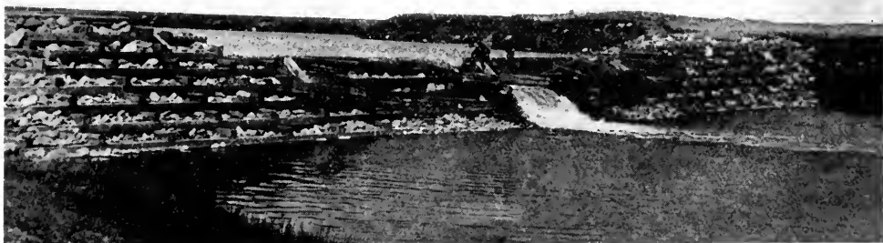
General view of rock-filled crib dam. This is a good type where timber and rock are plentiful. Photo shows the type of construction with square timber. Round timber notched out at the joints makes just as good a dam. This dam has a wood spillway, but the whole top can be made level and to act as a spillway. The water side of the dam has to be faced with planks or banked up with earth to stop leakage.
