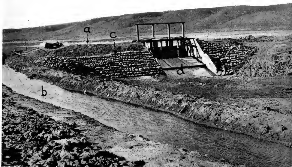
General view of earth dam. (a) Reservoir behind dam. (b) Ditch out of reservoir showing proper location for spillway channel around end of dam. (c) Rock riprap placed on dry side of dam to stop erosion by water running through wood spillway during floods. (d) Wood spillway through centre of dam. This shows the general idea but a straight drop is recommended. The height of the top of the dam above water surface in ditch represents the free board of the dam.
