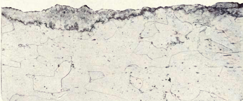
FIG. 31 — Section of sheet shown in Fig. 28, magnified 200 diameters, showing uneven tin coating and rough steel surface.
