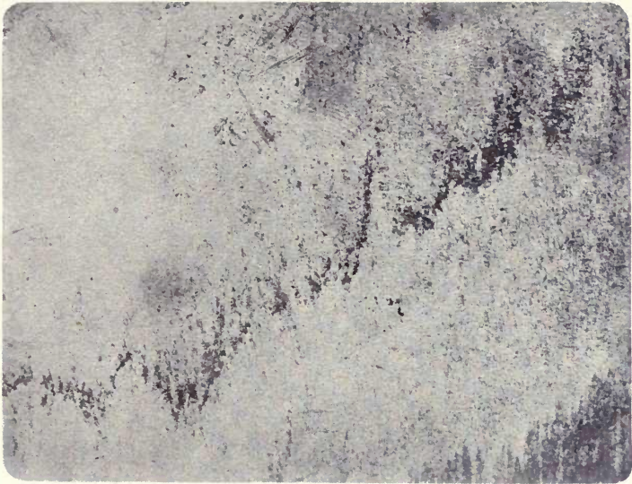
FIG. 22 — Natural size photograph of a black sheet showing mill scale on the surface.
