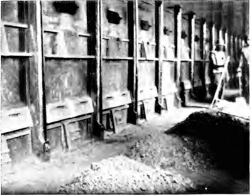
FIG. 1.—BATTERY OF PYRITES BURNERS.
