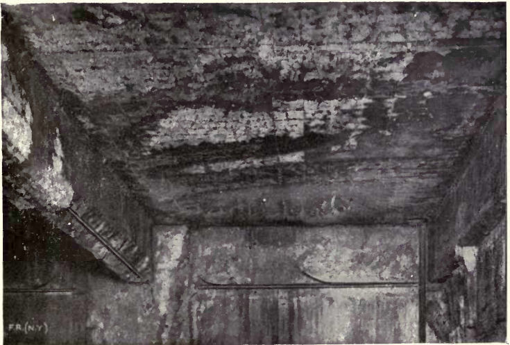
Fig. 10. —Effect of fire corner next to elevator in fourth story. Terra-cotta elevator partition has partially collapsed. Note spalled pilaster column and wall girders, also exposed reinforcement in floor slab.
