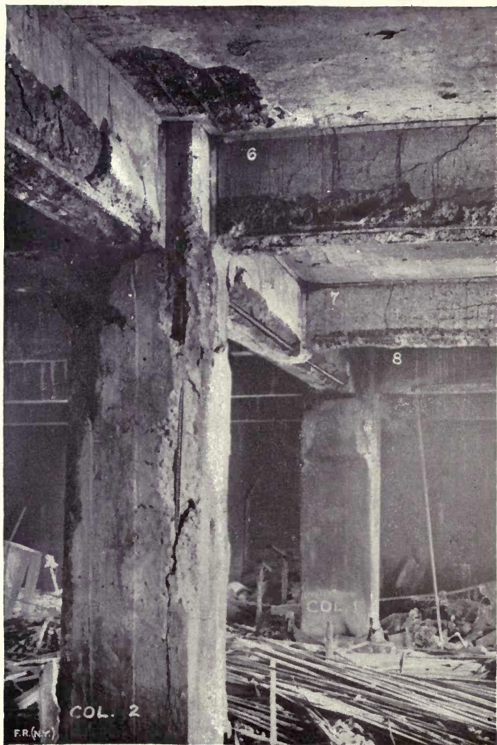
Fig. 8.—Looking eastward in third story, showing character of injury to concrete. Note unburned material on floor, also in Fig. 7.
