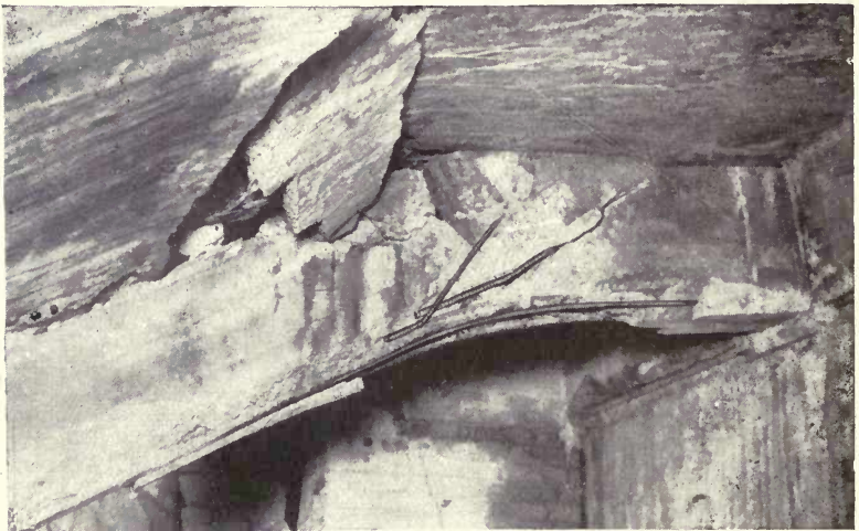
Connection of fallen beam No. 3 with wall girder in third story. (Figs. 5 and 6.)
