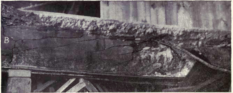
Girder Bin third story. The ribbed bar on the right belonged to fallen beam No. 3. The hole in bottom of girder is where the trussed bar pulled out.
