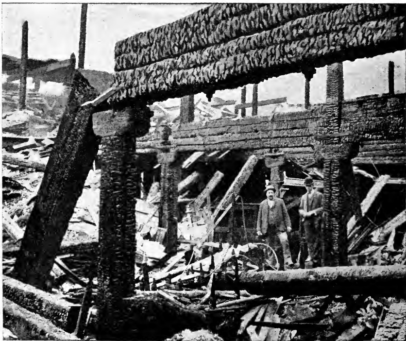
Fig. 14. What Is Left of a "Slow-Burning", "Mill-Constructed" Building after a Fire
