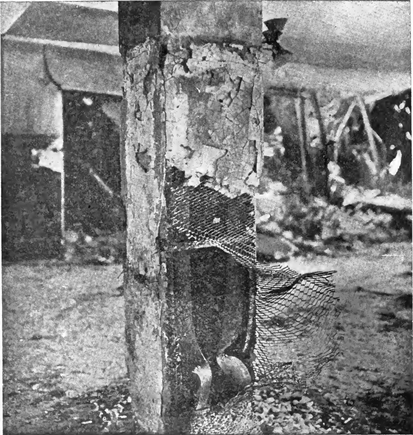
Fig. 2. A Wire and Plaster "Protection" to Steel Work
