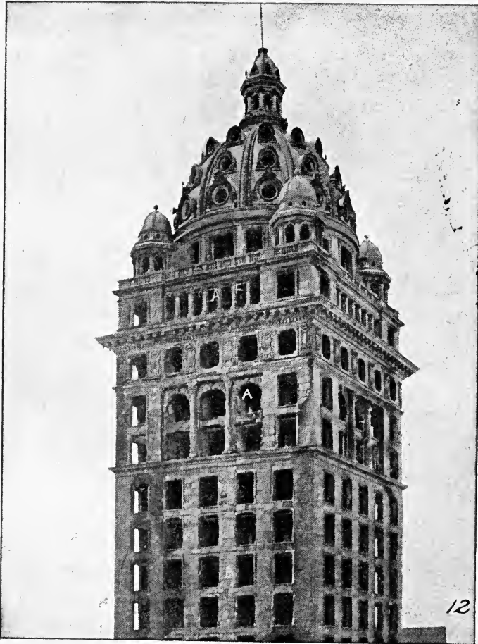
Fig. 39. Note Effect of a Fire Upon the Stone Work of the Upper Parts of a Tall Building
