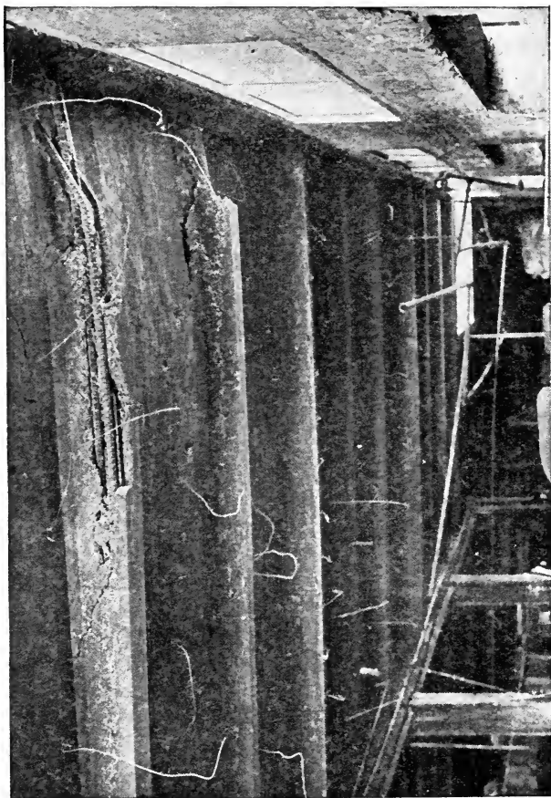
Fig. 6. Fire's Tendency to Expose and Distort the Reinforcement in Reinforced Concrete Work
