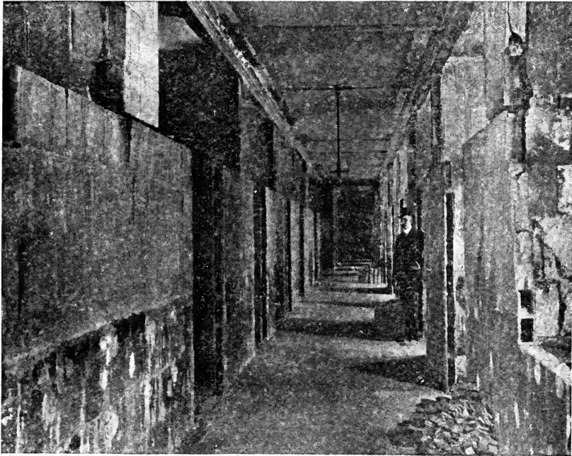
Fig. 3. Wooden Sash in Tile Partitions This construction permits fire to travel from room to room
