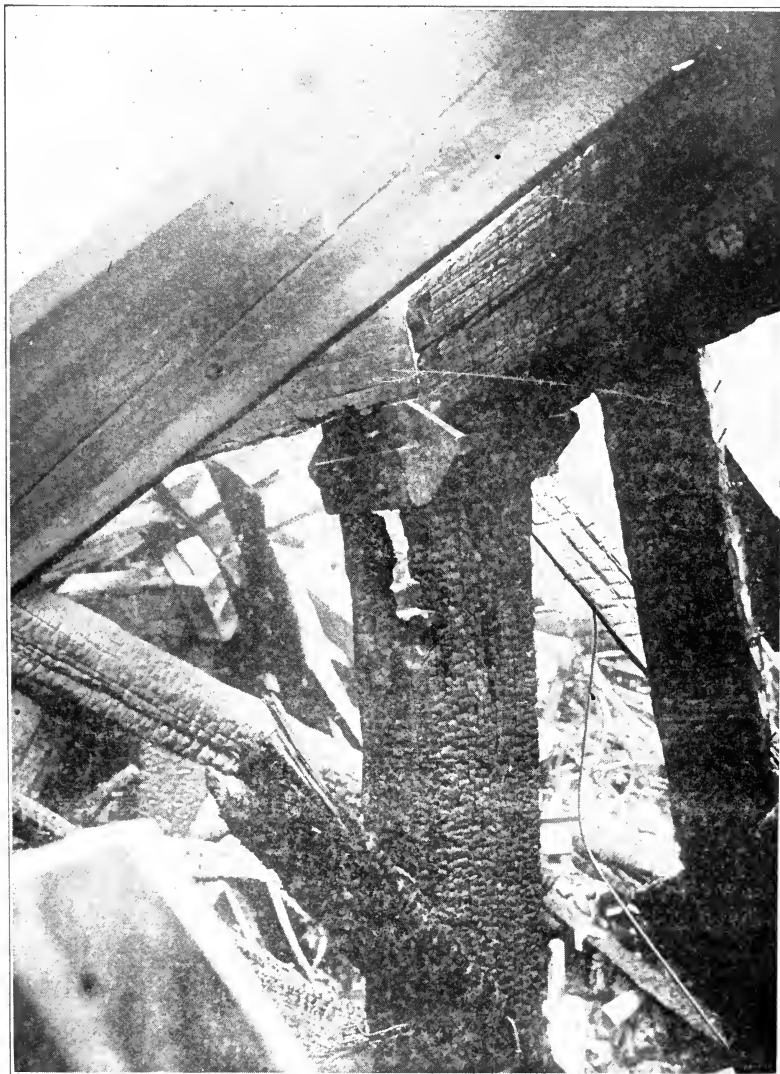
Fig. 72. "Slow-Burning" or "Mill Construction" After a Hot Fire, Utter Wreck
