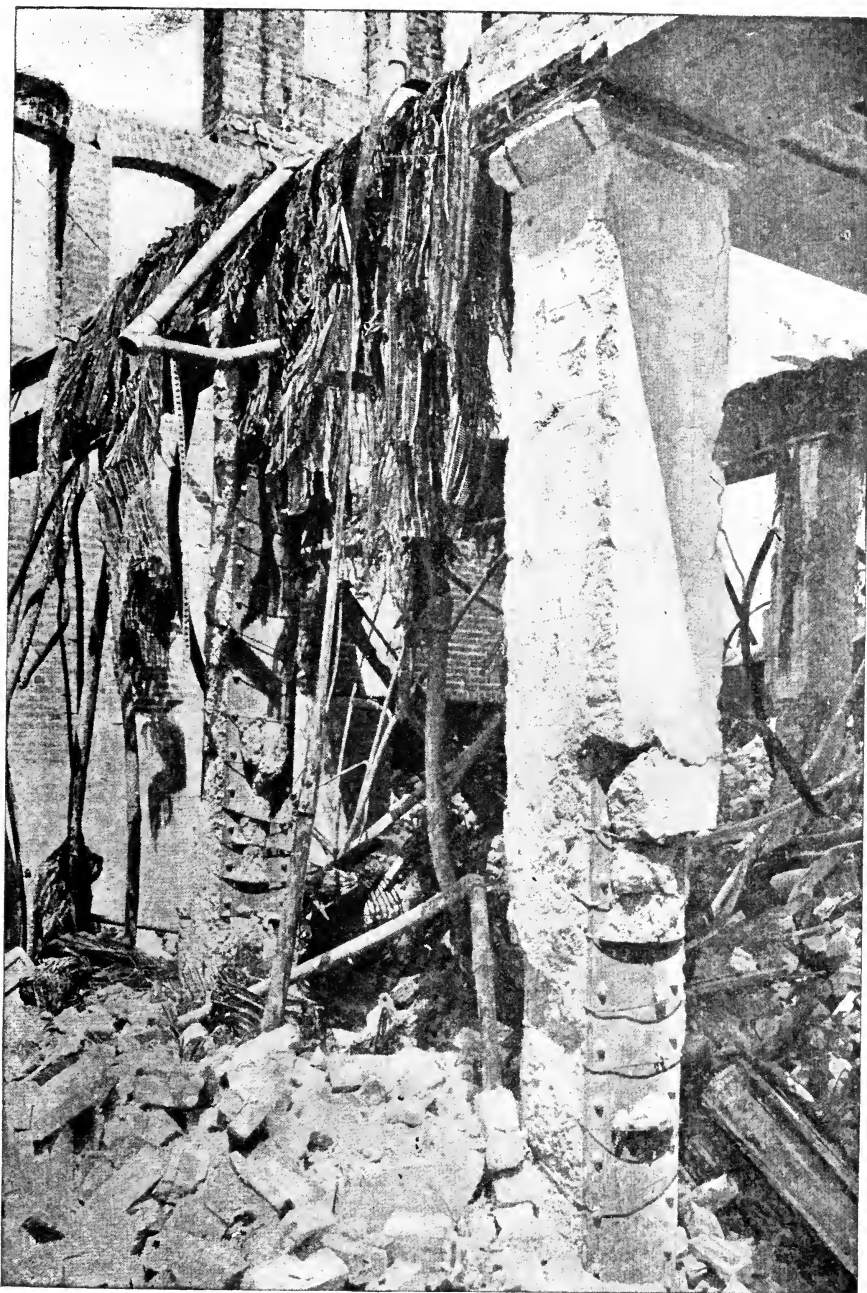
Fig. 25. Ineffective Fireproofing After a Fire
