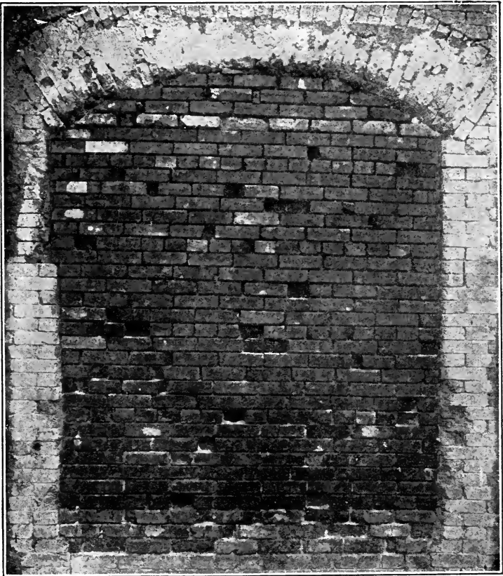
Fig. 112. Appearance of Test Panel of Brick After Exposure
