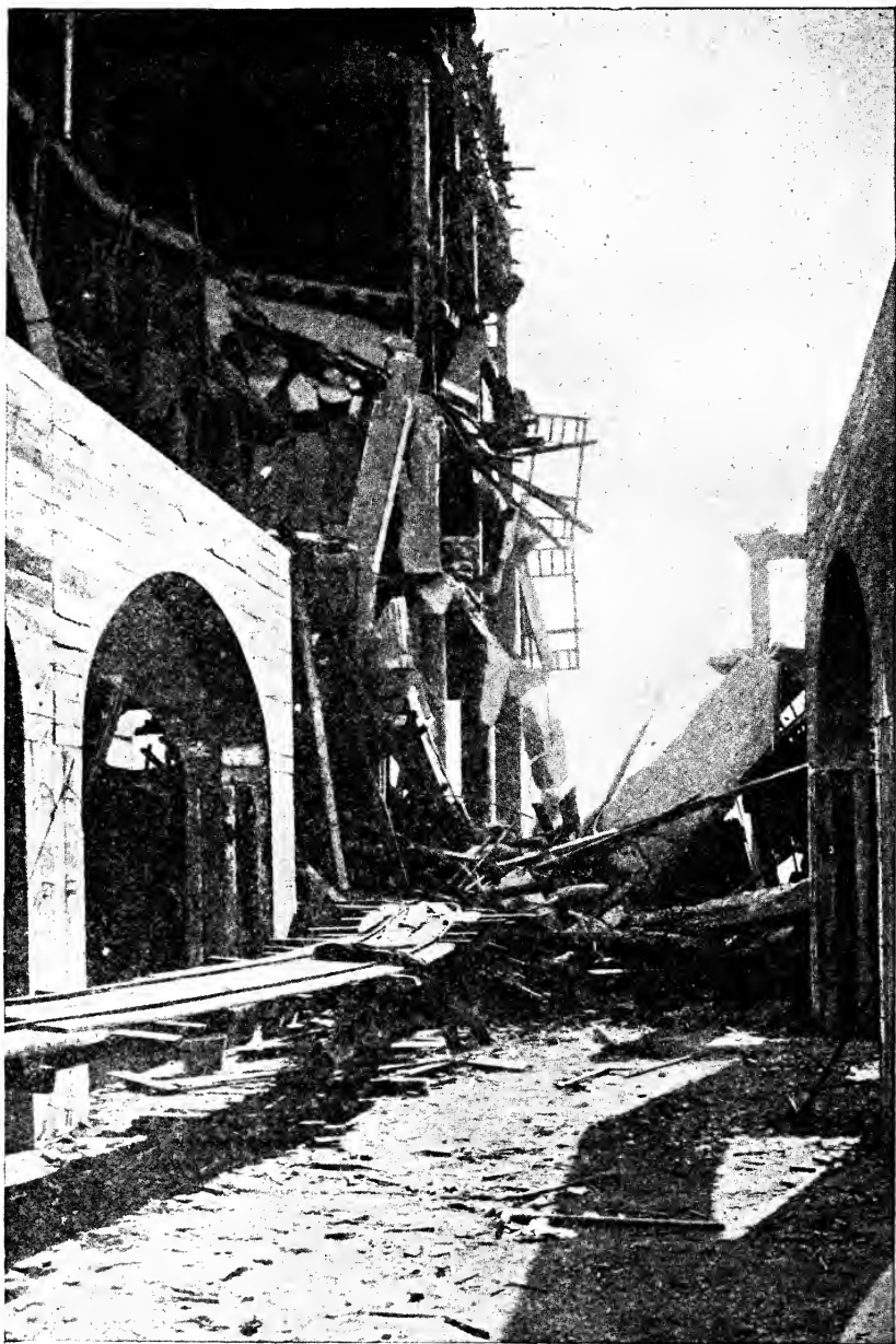
Fig. 36. The Bixby Hotel (California) Collapse, a Reinforced Concrete Structure
