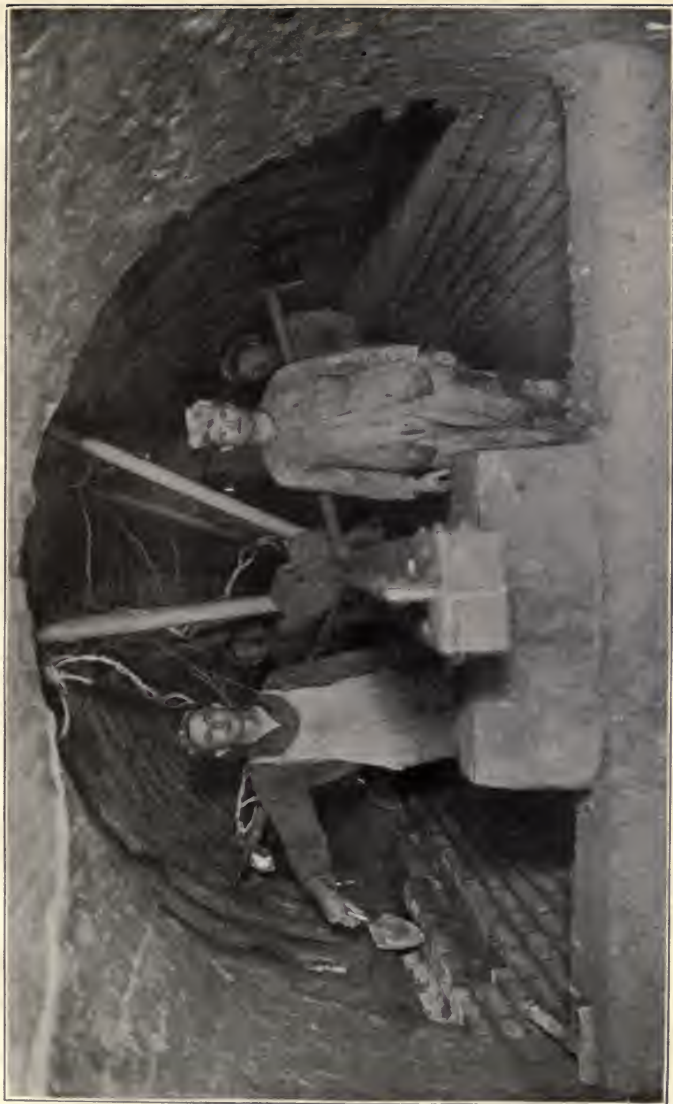
HEADING IN SEWER TUNNEL IN WEST ROXBURY BUILT IN QUICKSAND BY PNEUMATIC PROCESS.
