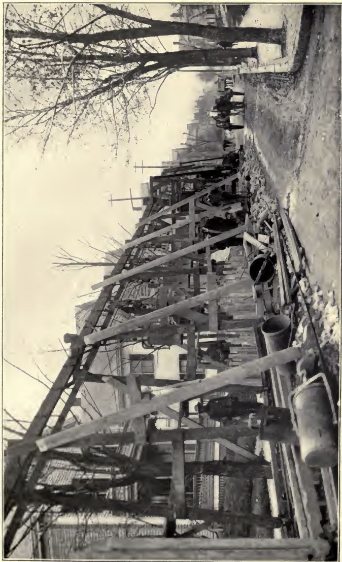
CONSTRUCTION OF SEWER BY USE OF EXCAVATING MACHINERY IN STREET IN MALDEN FOR EXTENSION OF NORTH METROPOLITAN SEWER.
