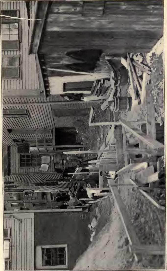
CONSTRUCTION OF SEWER TRENCH IN THICKLY SETTLED PART OF MALDEN FOR EXTENSION OF NORTH METROPOLITAN SEWER.
