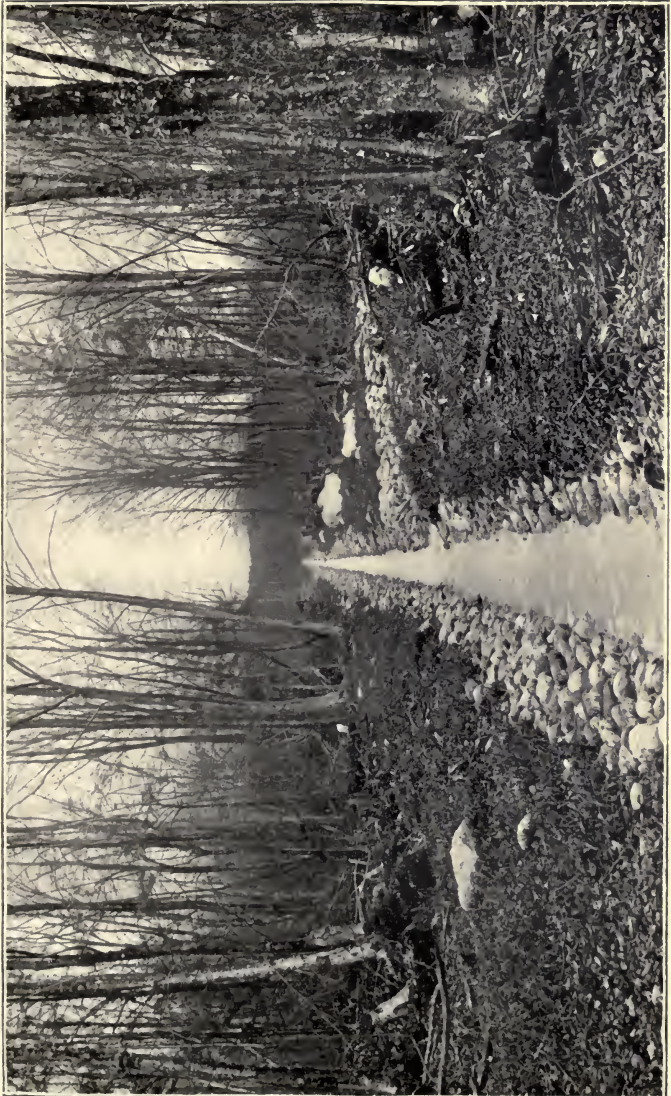
DITCHES FOR SWAMP DRAINAGE ON WACHUSETT WATERSHED IN HOLDEN.
