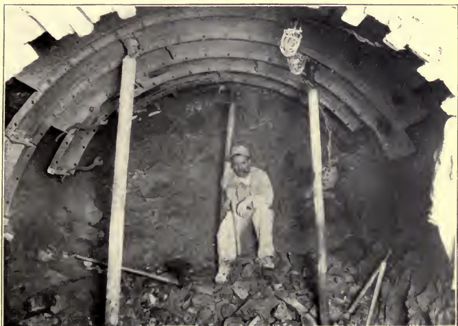
MYSTIC RIVER TUNNEL EXTENSION — HEADING IN ROCK IN TUNNEL UNDER THE RIVER.
