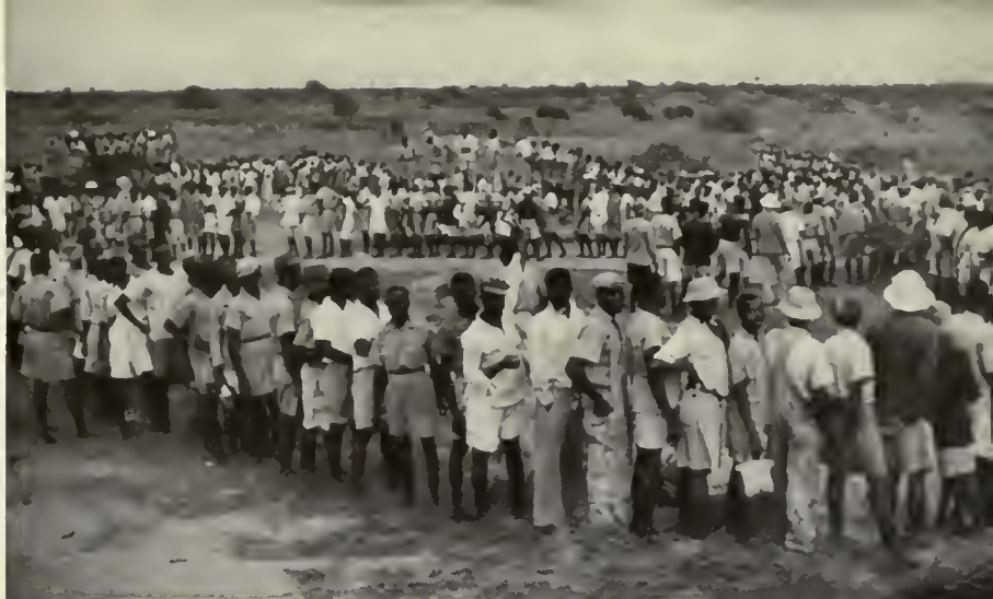
▲ Five o'clock line-up at end of day's work. Army trucks carry laborers from base to city. (below) Modern installations built with ancient construction methods.
