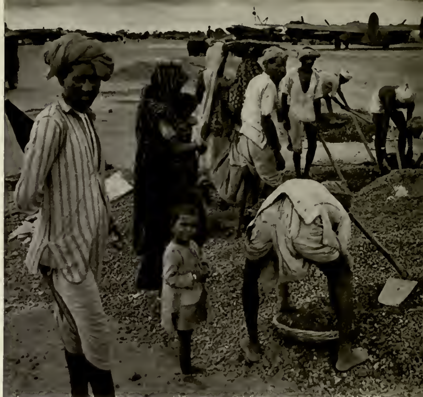
ATC AIRPORTS ARE CONSTRUCTED BY PRIMITIVE METHODS AND SHEER NUMBERS OF LABORERS
