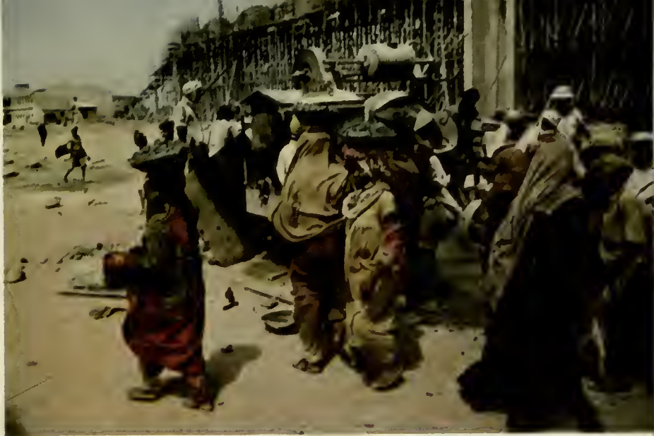
Airport construction in India. From cement mixer hundreds of women, robed in gay colors, carry concrete via head pans to end of runway, half mile distant.
