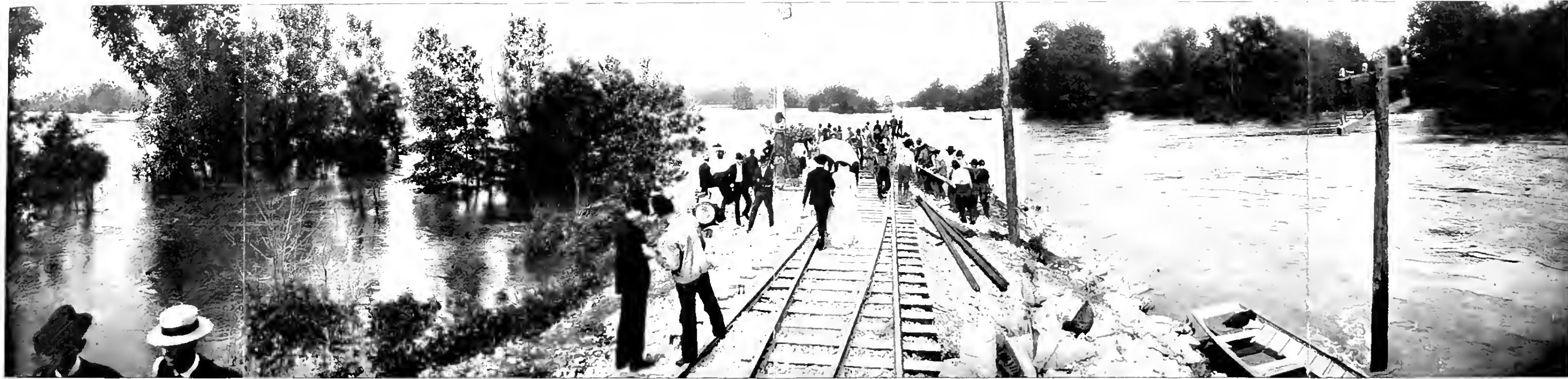
View of the bridge over the river and M. showing break in track of 80 feet where the water rushed through to a depth of 20 feet.
