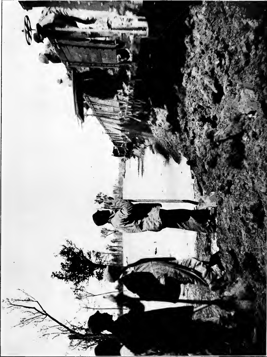
FIG. 6.—CLOSING BEULAH CREVASSE. Dumping dirt on river side of rock fill, March, 1913.
