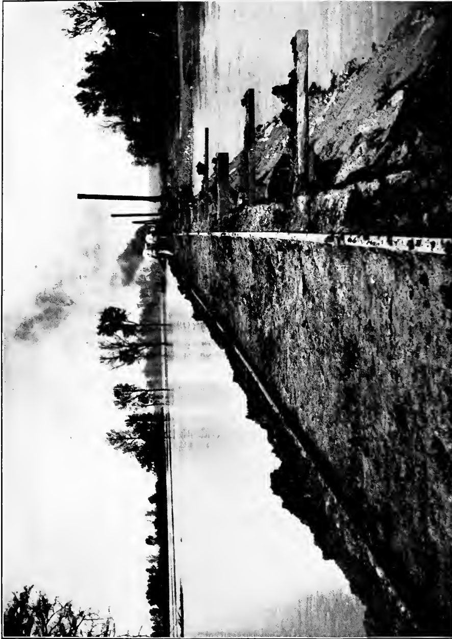
FIG. 8.—CLOSING BEULAH CREVASSE. Both sides of fill. Note difference in height of water. 1913.
