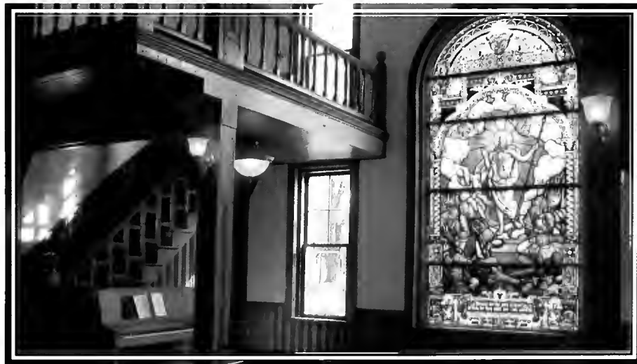
Inside the CCM, walls were re-plastered. Wood work that was missing or damaged by water leaks was replaced by oak trees salvaged from the College Woods.
