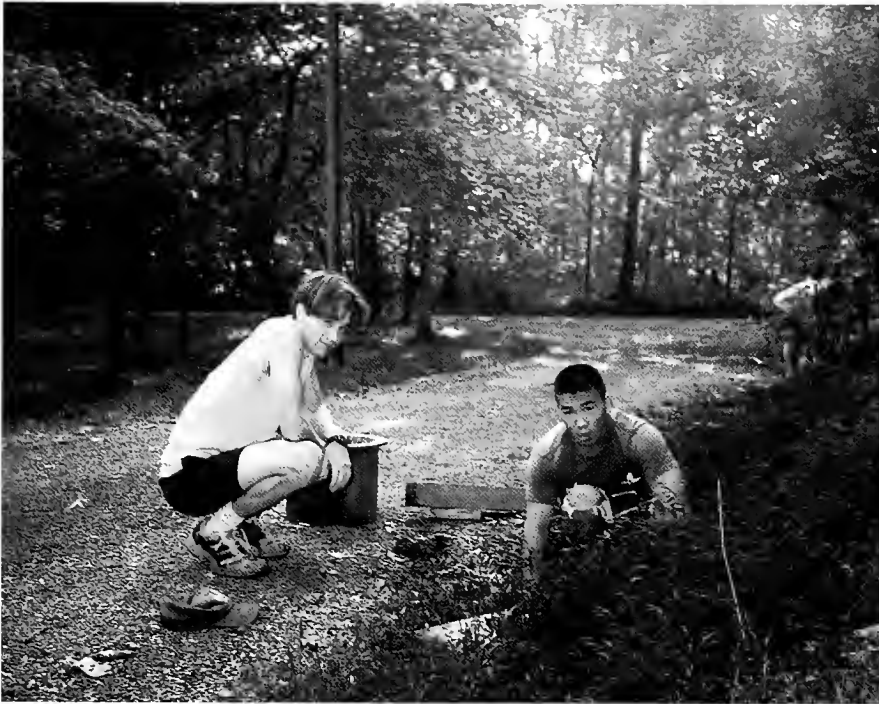
Juniors Lanny Blackwood and Kimiaki Itamura, both Bonner Scholars, work to replace a culvert at Camp John Knox. This was the second year that the Bonner Scholars have used the camp for fall orientation.
