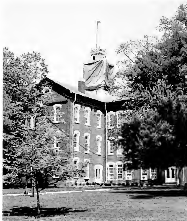
Anderson Hall under wraps ... The College continued work on deferred maintenance and renovation projects this year, including cleaning and painting the exteriors of Anderson and Fayerweather Halls, restoration of most residence halls and the renovation of the third floor of Fayerweather to provide critical office space.
