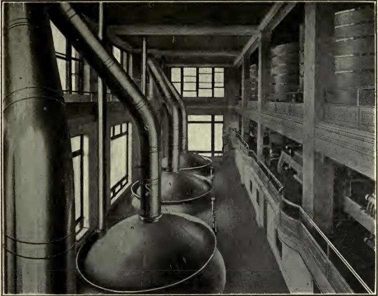
Fig. 78.—Copper Boilers. (Courtesy of the United States Brewers' Association.)
