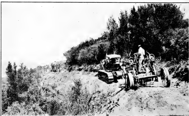
The latest type of machinery is used in building national-forest roads and trails
