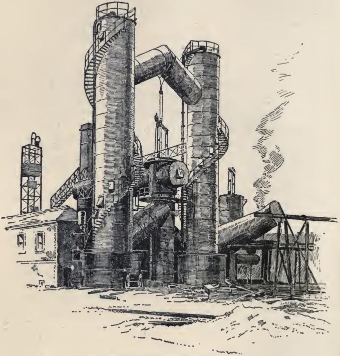
Fig. 55.—Ammonia Condensers, Langloan.
