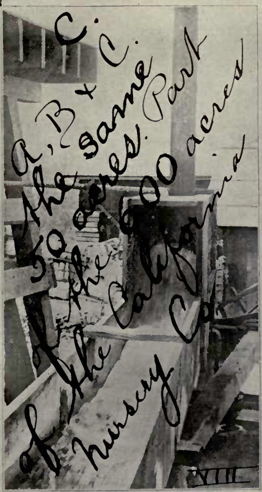
AT THE PUMPING PLANT OF THE NILES STRAWBERRY FARM Fifteen-horsepower electric motor; 700 gallons per minute.
