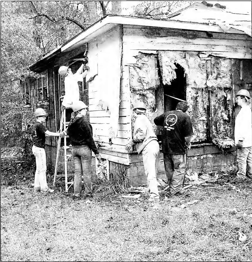
Students and staff members from the University of North Carolina at Chapel Hill are seen working on the exterior of a house in the North Carolina State University area. The house is in need of significant repairs and is being prepared for occupancy by a family of four. The students and staff are working on the exterior of the house, which is in need of significant repairs. The house is being prepared for occupancy by a family of four. The students and staff are working on the exterior of the house, which is in need of significant repairs. The house is being prepared for occupancy by a family of four.
