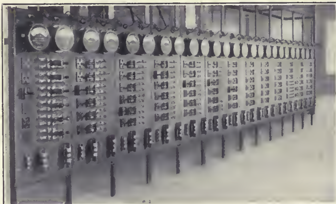
Switchboard Built By Us To Charge 78 Vehicles At One Time
