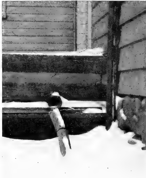
This pipe drains a kitchen sink and sub-irrigates a flower bed
