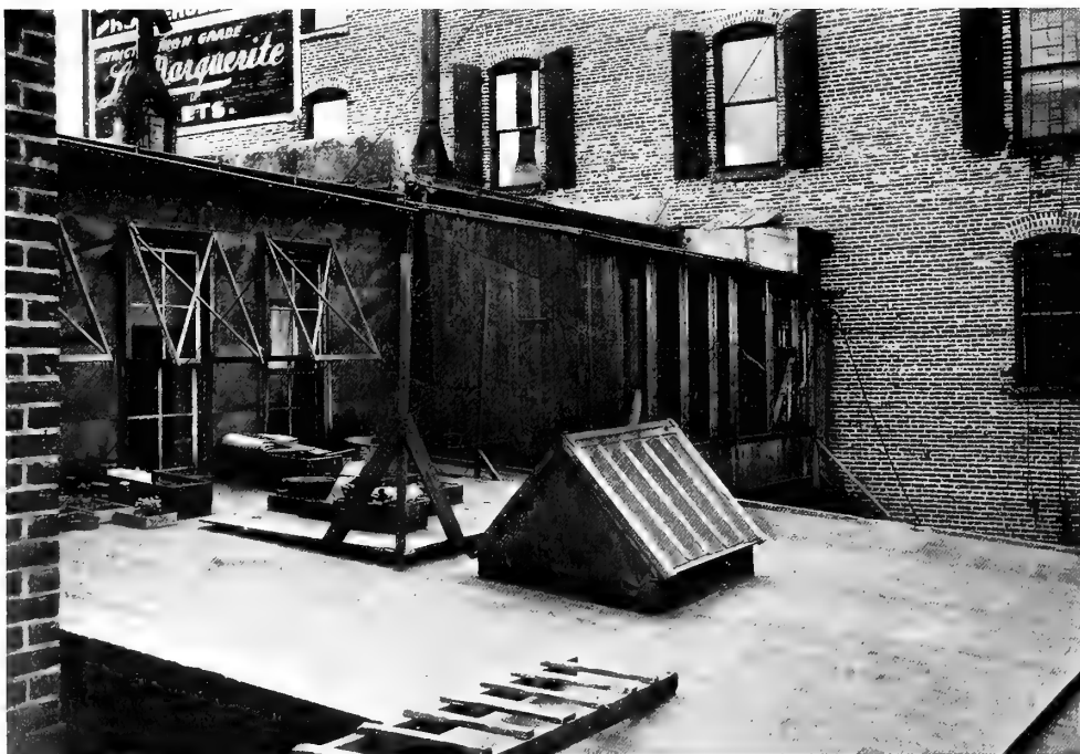
A bare, unsightly place which radiated so much heat as to make the adjoining rooms unendurable
