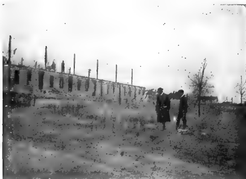
TEARING DOWN BUILDINGS AT GARDEN CITY, L. I., WHERE NEW PLANT WILL BE
