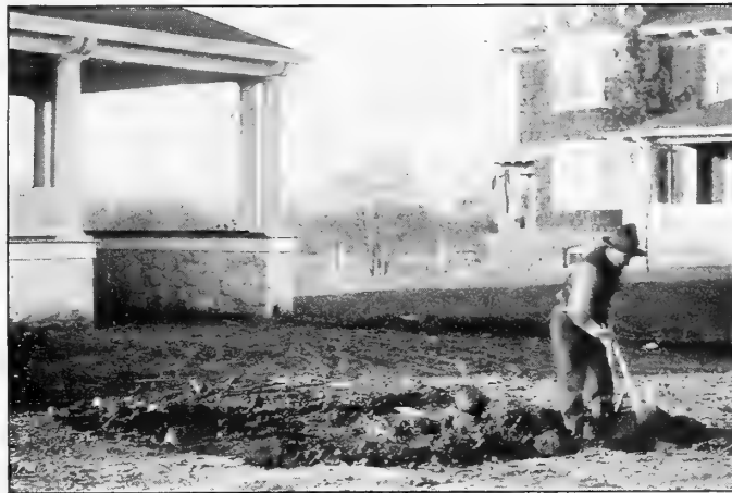
A good start is essential. Be sure that the soil from the cellar is not left around on the surface. Either remove it or cover with good top soil
