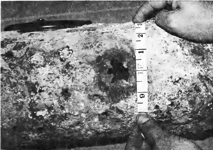
Figure 7. Corrosion hole in the pipe.
