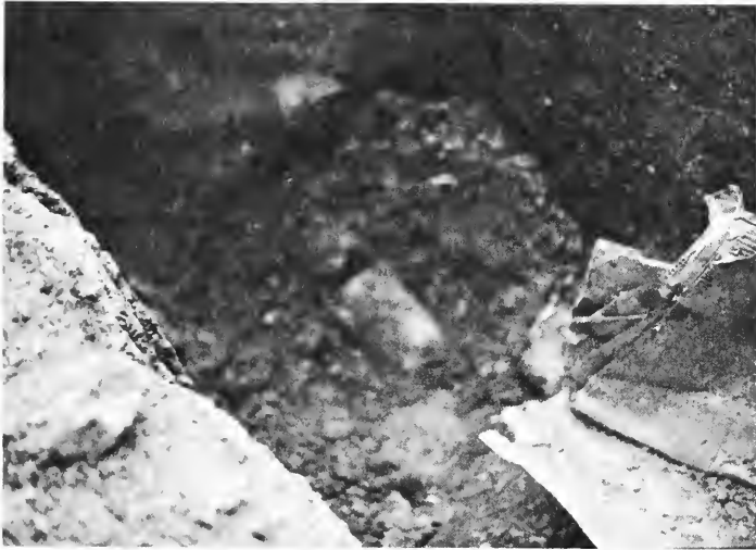
Figure 6. Broken sewerline below corrosion hole leak.
