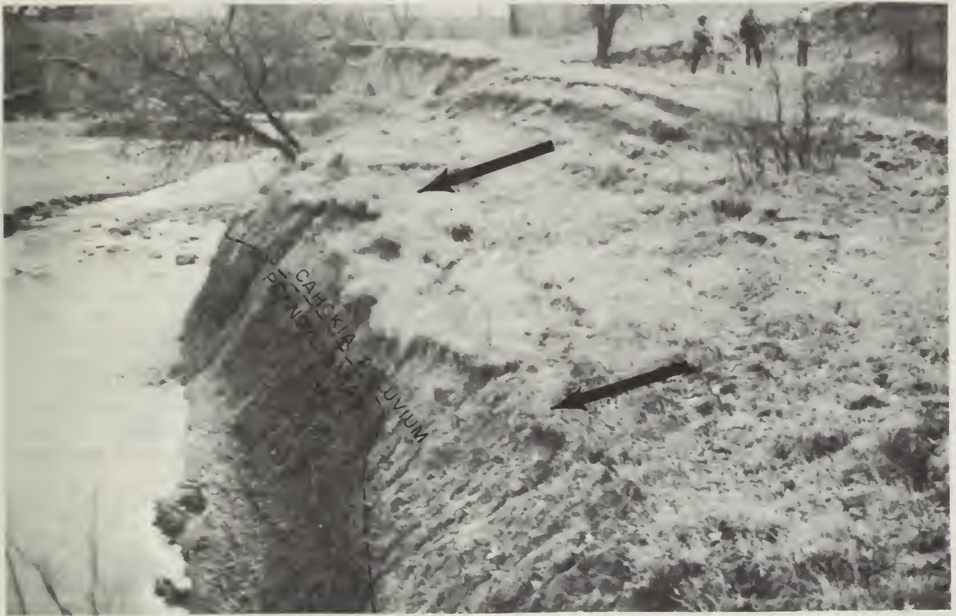
Figure 12. Cut bank along Case Creek, SE¼ NE¼ Sec. 30, T. 17 N., R. 1 W., Rock Island County, showing Lacon Formation (slump). The slump consists of recognizable Cahokia Alluvium and Pennsylvanian shale. The entire block extending from the foreground to the scar just beyond the figures in the upper right has moved toward the creek and has broken into numerous smaller pieces. Arrows show movement of the block. Photo taken December 20, 1971.
