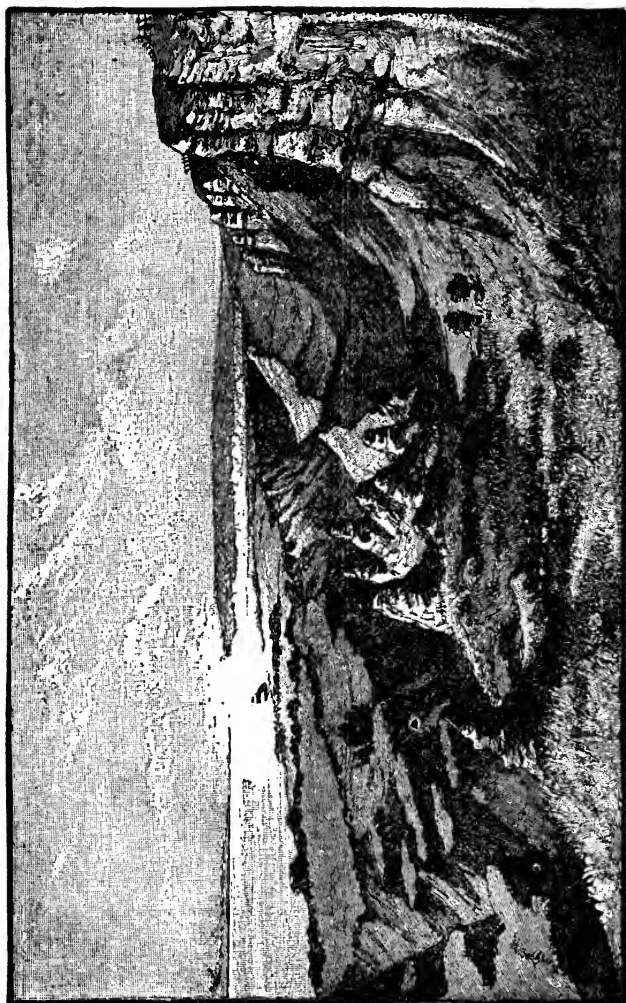
FIG. 18.—VIEW OF AXMOUTH LANDSLIP (AS IT APPEARED IN APRIL 1885).
