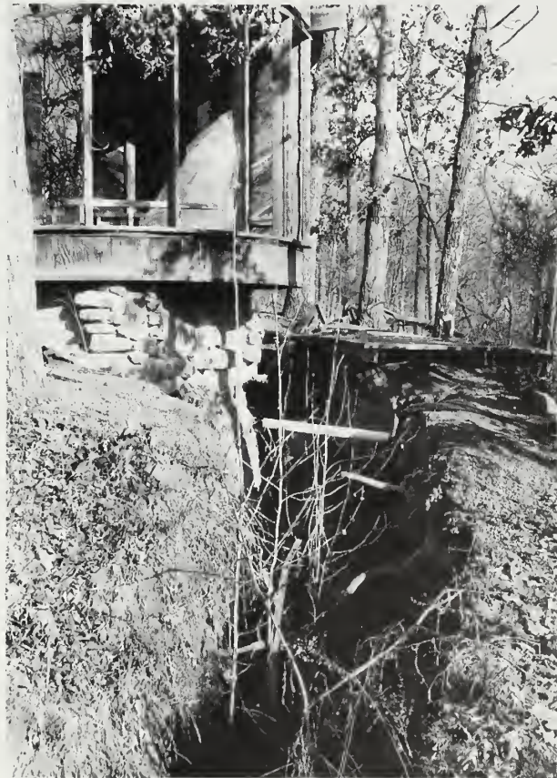
Figure 23 Tension fissure caused by a landslide on the north side of Grassy Creek. The creek is to the south (right) of the house.
