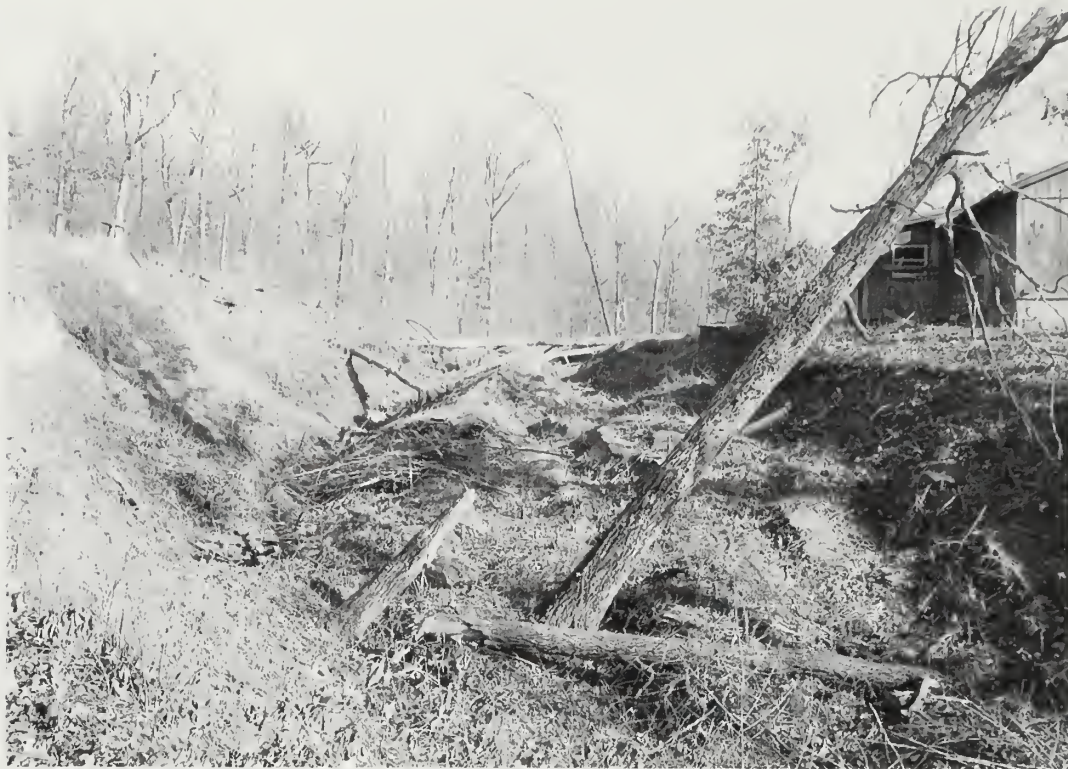
Figure 24 A graben created by a landslide on the north side of Grassy Creek. The view is to the east; the house to the right is the same house shown in figure 23. The scarp on the uphill side (left) apparently is the major glide plane of the landslide, whereas the scarp to the right represents an antithetic fault. The hazards of building on steep slopes underlain by the Glasford Formation are evident in this photo.
