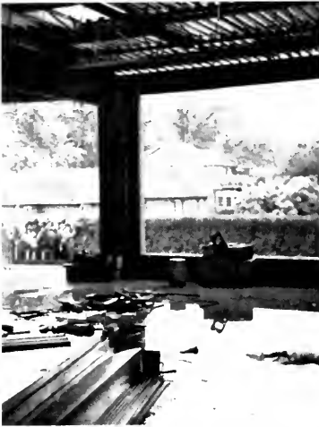
Library after air-conditioning was installed!
