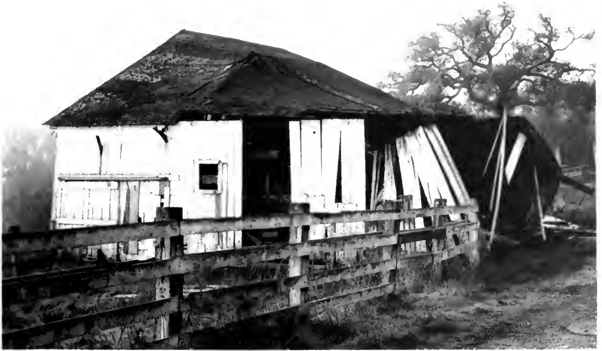
The horse barn shortly before it was demolished, February 1994. NPS photograph by Dewey Livingston.
