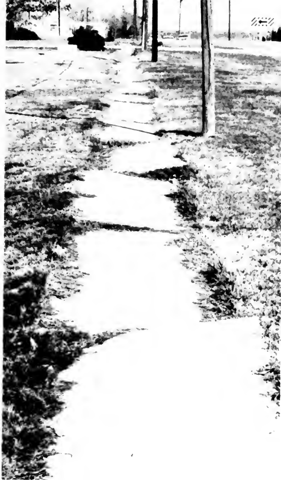
Sidewalk damage from clayey soil with high shrink-swell potential. Soils of this type have same effect on basement walls and floors.
