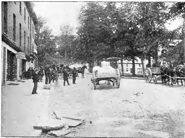
View on High Street, Brattleboro, Vt., looking from Main Street, showing teams hauling crushed stone, and road roller at work. Governor Fuller is seen near the centre of the picture in consultation with Road Commissioner Eames.
