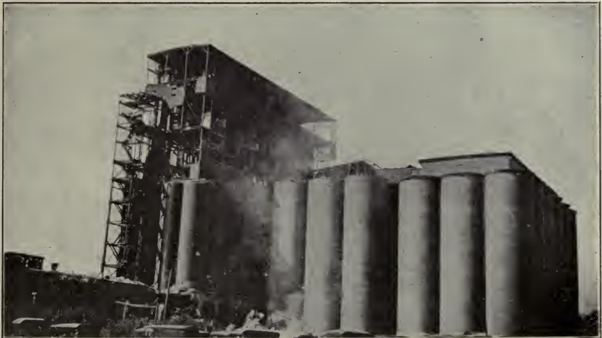
FIG. 13.—Explosion traveled from basement through man-lift tower to "texas" or top of elevator.
