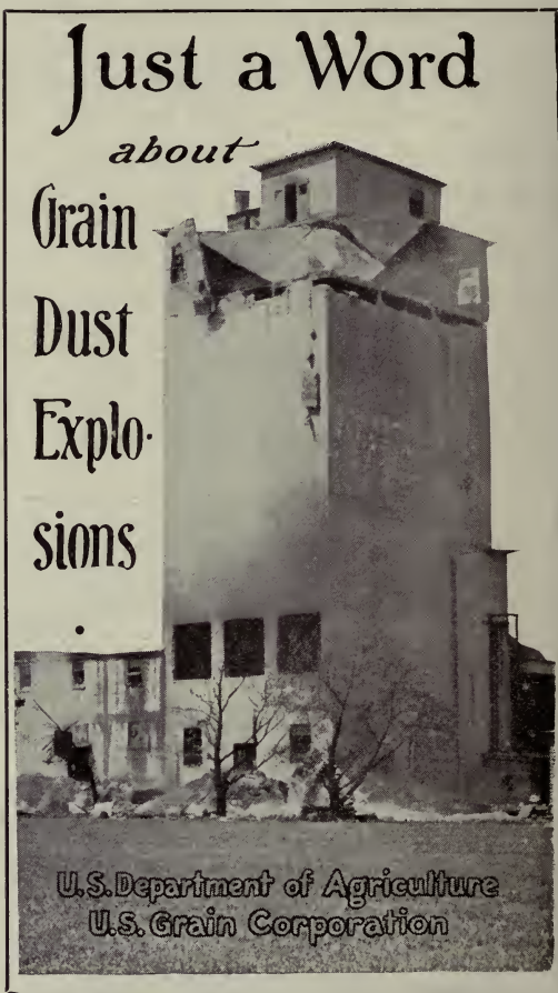
FIG. 7.—Upper portion of this plant destroyed by dust explosion. From cover-page of pamphlet used in educational campaign.
