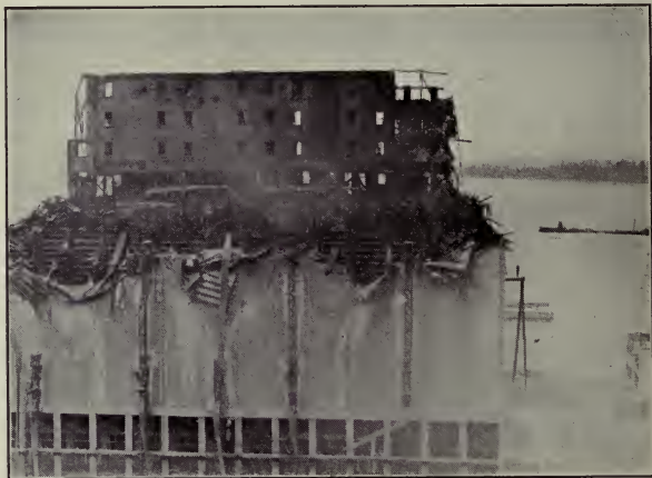
FIG. 11.—Upper portion of grain elevator badly damaged by dust explosion. Note "trough-like" construction of interior walls of bins.
