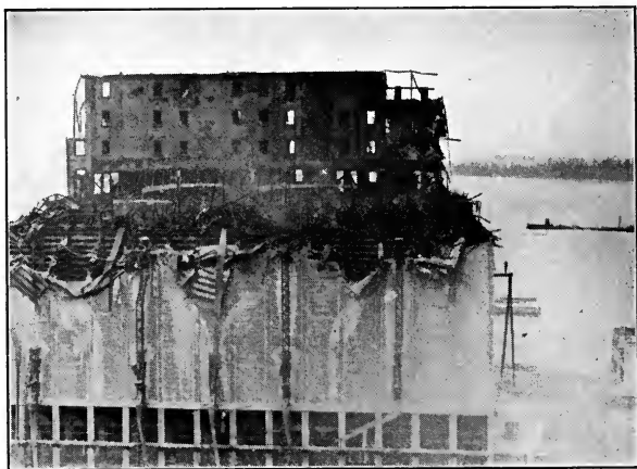
FIG. 11.—Upper portion of grain elevator badly damaged by dust explosion. Note "trough-like" construction of interior walls of bins.
