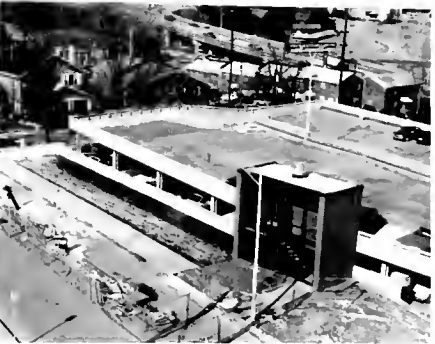
above: This series of photos taken from the 2nd floor at the north end of the Hanes Building shows the razing of 3 houses (1 not seen) on Beach Street and the removal of a 26-car parking lot to make room for the expansion of the Eden Terrace parking deck.
