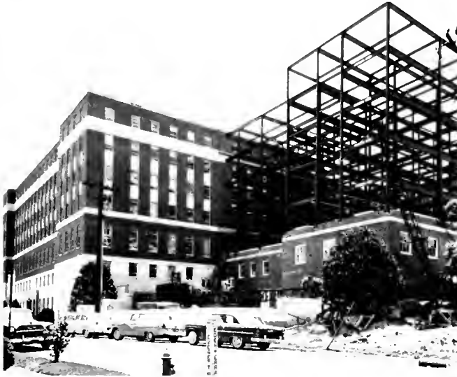
above: The Research Building and the Vivarium Extension under construction, on the west end of the medical school, are shown here around 1961.
