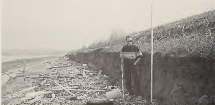
28 Randolph County: Nearly vertical cut made by waves eroding the inner (landward) side of the southern part of the Kaskaskia Island levee. Note the driftwood and debris where IGS engineering geologist, Robert Bauer, stands at the base of the erosional cut (October 13, 1993).
