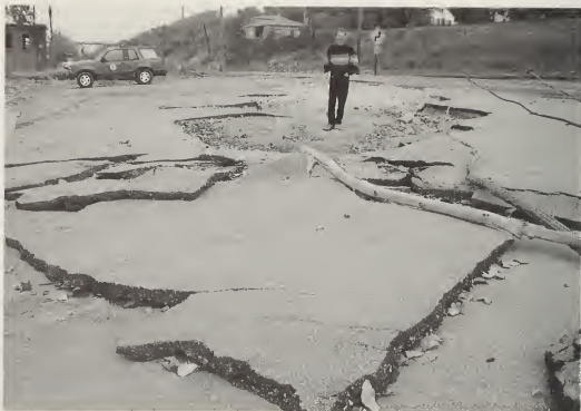
4 Randolph County: Asphalt pavement slabs next to the river-front road at Chester were lifted and transported by flood water. Robert Bauer, ISGS engineering geologist, stands where the blacktop slabs were eroded (October 13, 1993).
