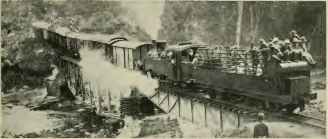
Reconstructed after Demolition by the Germans: testing a bridge on the Northern Cameroon Railway with a heavily loaded train
