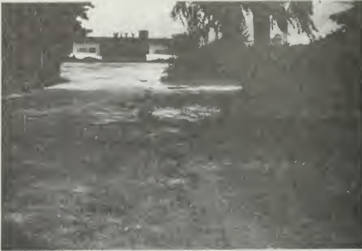
8a. Severe cracking of asphalt driveway. House to right was so severely damaged that it was torn down. (DuMontelle, 1967.)
