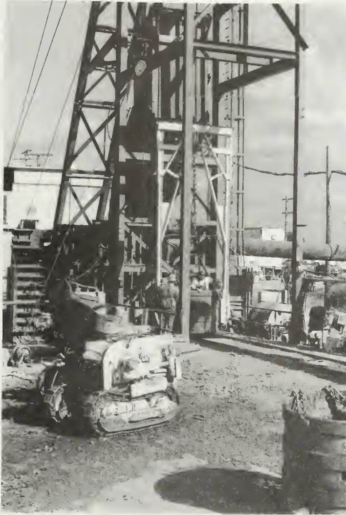
Figure 28 Construction site of new mine air shaft for Amax Coal Company, Wabash Mine (photo by W.T. Frankie).
