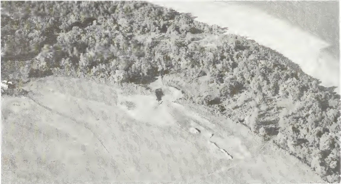
Figure 34 Site failure of the Denham Levee was caused when flood waters crested the levee in the spring of 1996. This failure created a large circular scour at the base of the levee (photo by W.T. Frankie).
