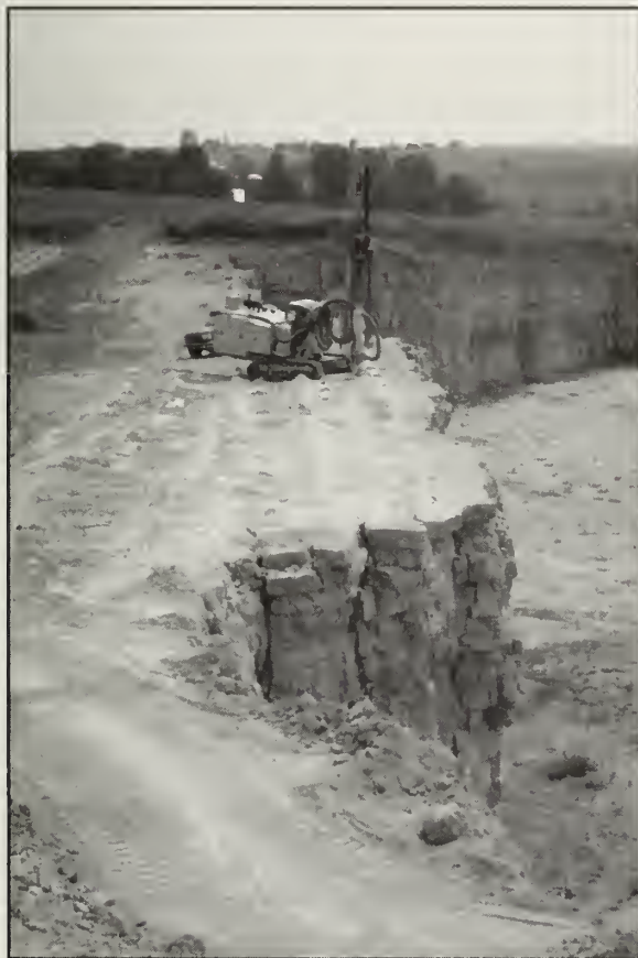
Figure 24 Drilling operation on the upper bench at Youngbluth Quarry, preparing for a shot (photo by W. T. Frankie).
