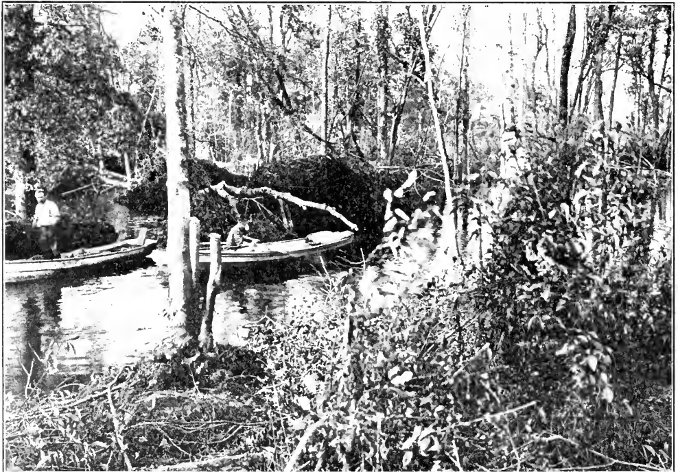
THE MEN GO OUT IN BOATS TO ATTACH A WIRE CABLE TO THE STUMPS.
