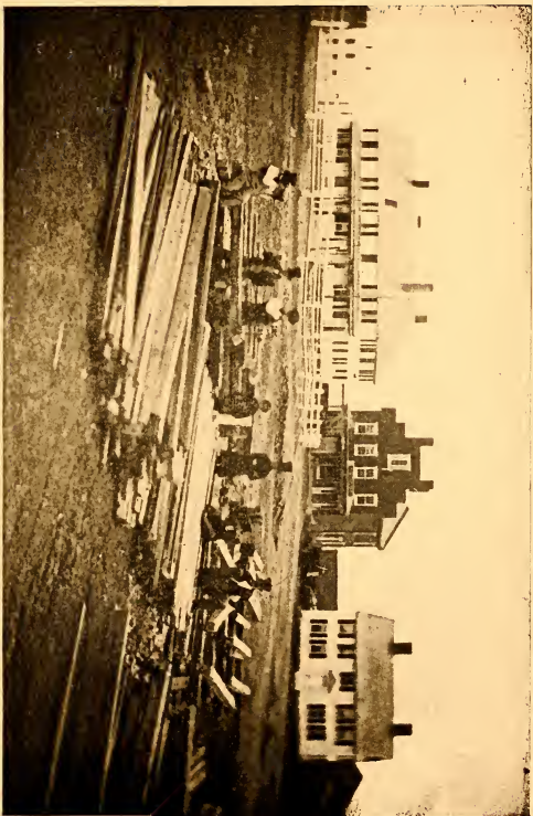
BUILDING THE NEW TOWN HOUSE IN 1854. Old Leicester Hotel background at left.
