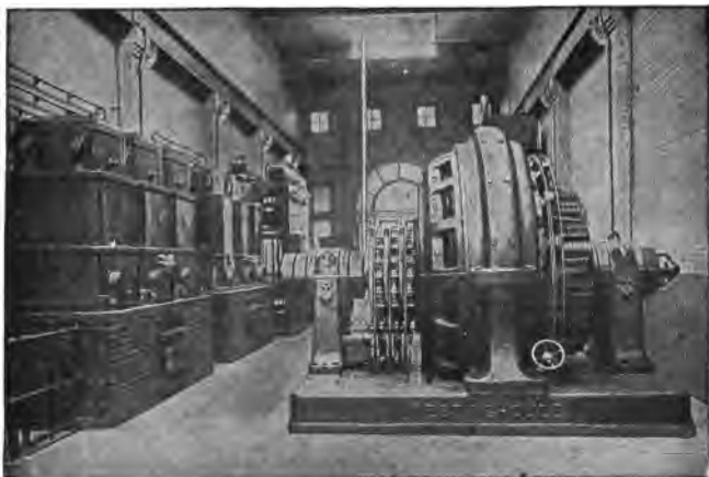
FIG. 2,198.—Example of converter sub-station, showing the Brooklyn Edison Co. Madison sub-station. The transformers are seen on the left, the converter shown at the right is a Westinghouse synchronous booster rotary converter, consisting of a standard rotary converter in combination with a revolving armature alternator mounted on the same shaft with the converter and having the same number of pole. The function of the machine is to convert and regulate the pressure. By varying the field excitation of the alternator, the A.C. voltage impressed on the rotary converter proper can be increased or decreased as desired. Thus, the D.C. voltage delivered by the converter is varied accordingly. This type of converter is well adapted for any application for which a relatively wide variation, either automatic or non-automatic, in direct current voltage is necessary. Also especially for serving incandescent lighting systems where considerable voltage variation is required for the compensation of drop in long feeders, for operation in parallel with storage batteries and for electrolytic work where extreme variations in voltage are required by changes in the resistance of the electrolytic cells.
