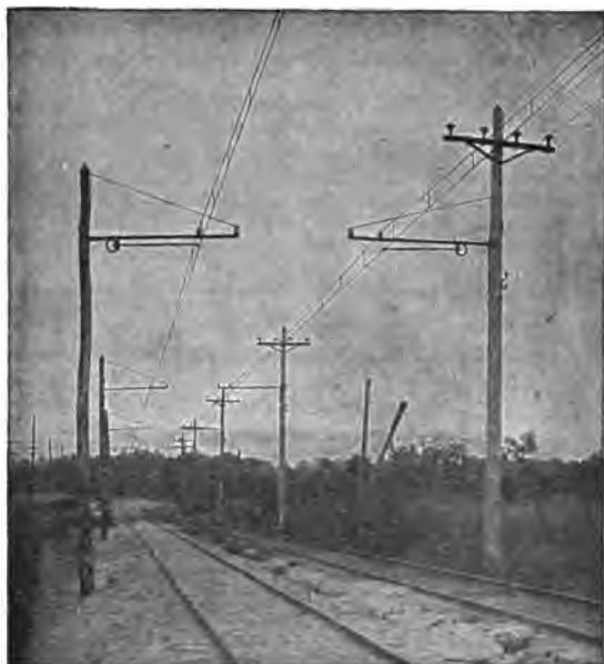
FIG. 2.135.—Typical American overhead 6,600 volt single phase interurban trolley line, Baltimore and Annapolis short line, Annapolis, Md.
