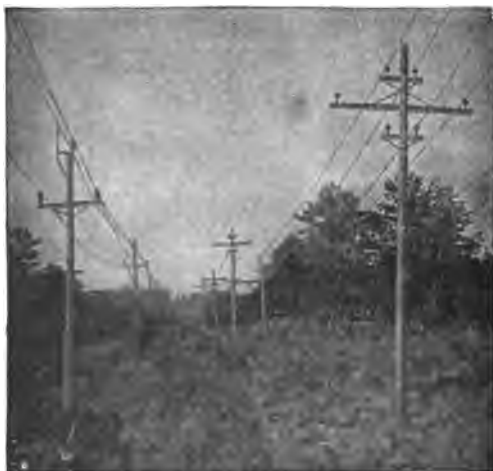
FIG. 2,142. —Single and twin circuit poles (Southern Power Co.). The twin circuit pole at the right is used for 11,000 volt circuits, while the single circuit poles at the left carry 44,000 volt conductors, being used on another division for 100,000 volt line.
