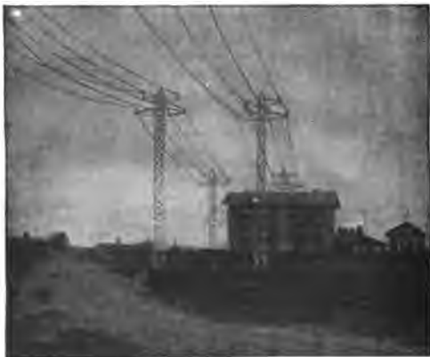
FIG. 2,138.—44,000 volt lines entering the Gastonia sub-station of the Southern Power Co. The poles used are of the twin circuit two arm type, built of structural steel, their height varying from 45 to 80 feet, the latter weighing 9,000 pounds each. These poles have their bases weighted with concrete.
