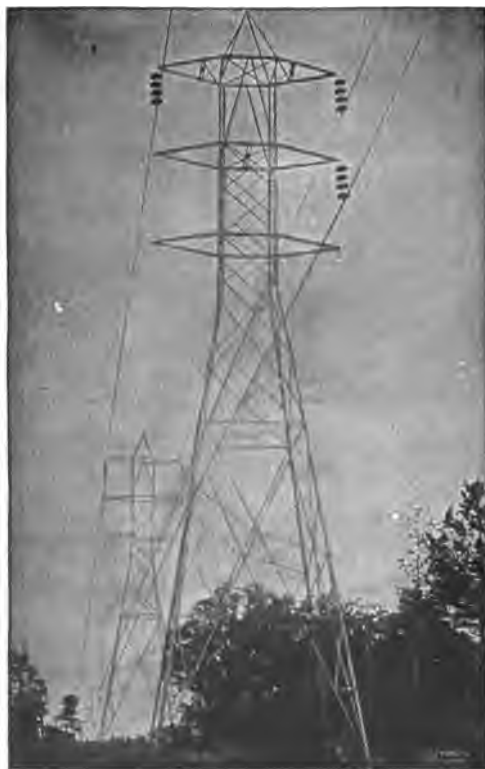
FIG. 2,144.—100,000 volt "Milliken" towers with one circuit strung (Southern Power Co.). These towers are mounted on metal stubs sunk 6 feet in the ground. Where the angle of the line is over 15 degrees, however, these stubs are weighted with rock and concrete, and where an angle of over 30 degrees occurs, two and sometimes three towers are used for making the turn. The weight of the standard "Milliken" tower is 3,080 lbs., and its height from the ground to peak is 51 feet. The towers are spaced to average eight to a mile and a strain tower weighing 4,250 lbs. is used every mile. For particularly long spans a special heavy tower weighing 6,000 lbs. is used. The circuits are transposed every 30 miles. Multiple disc insulators are used, four discs being used to suspend each conductor from standard towers and ten discs to each conductor on strain towers. The standard span is 600 feet, sag 11 ft. at 50° Fahr.
