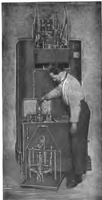
FIG. 2.119. —General Electric series mercury arc rectifier outfit; view showing method of replacing a tube. The illustration also shows tube carrier and drip tray.
