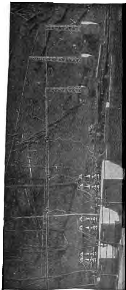
FIG. 2,174.—View from roof of power house of the Schaghticoke-Schenectady transmission line, showing anchor poles, strain insulators, lightning arrester horn gap and line entrance bushings.
