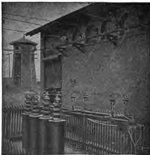
FIG. 2,397.—Highland Park sub-station, Charlotte, N. C., showing old lightning arrester tower on the left and General Electric aluminum (electrolytic) cell lightning arrester and horn gaps in foreground.
