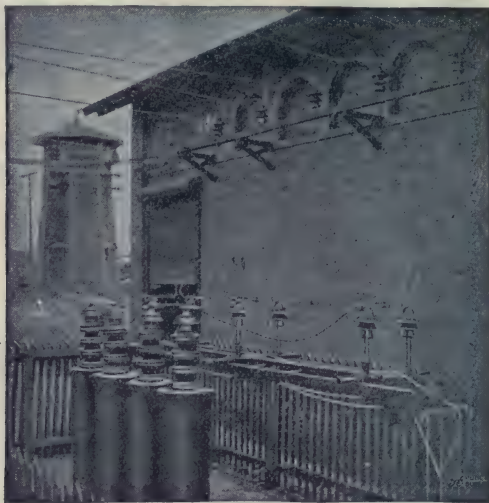
FIG. 2,397. —Highland Park sub-station, Charlotte, N. C., showing old lightning arrester tower on the left and General Electric aluminum (electrolytic) cell lightning arrester and horn gaps in foreground.
