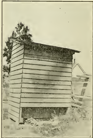
FIG. 7. A good privy building which is capable of reconstruction to meet the requirements for improved privies.
